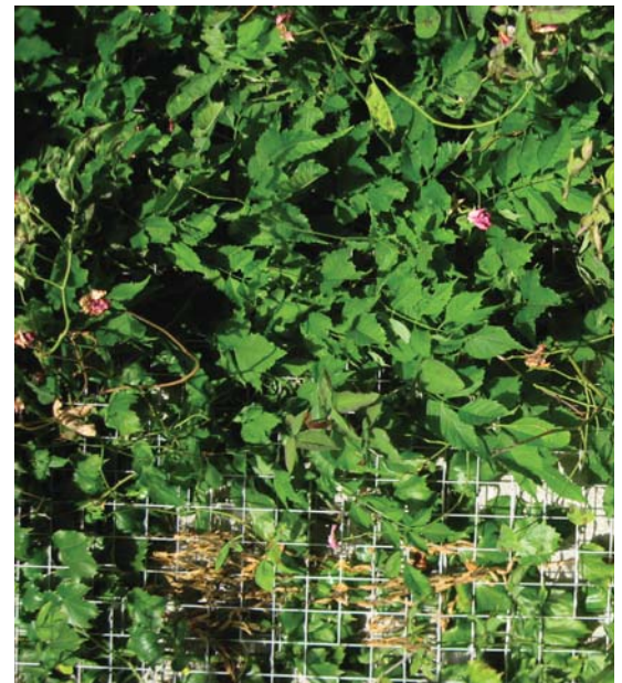
Green walls are becoming a common language on the campus, increasing greenery where large blank walls occur
